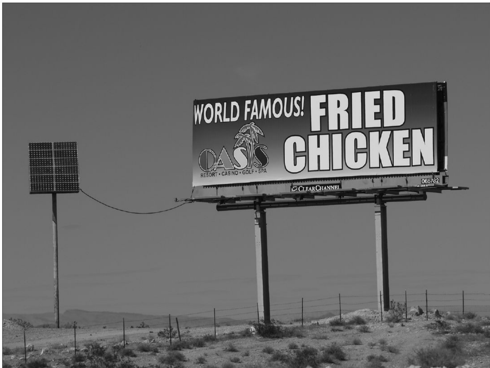
Pole-mounted panels powering billboard lights.
